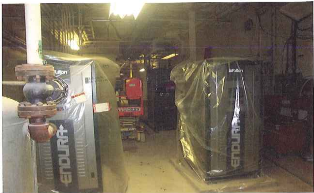
MAIN CTE BUILDING – MECHANICAL ROOM – DECEMBER 2013
