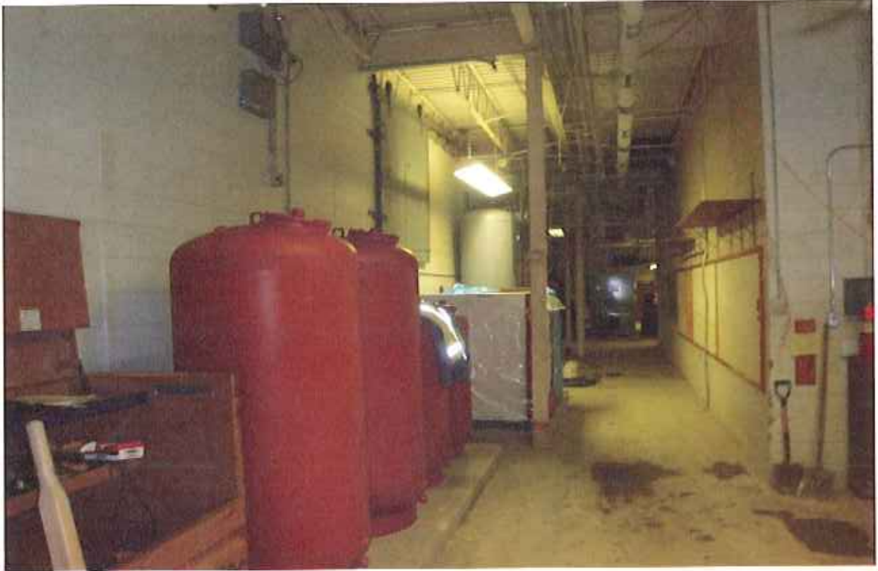
MAIN CTE BUILDING – MECHANICAL ROOM – DECEMBER 2013
